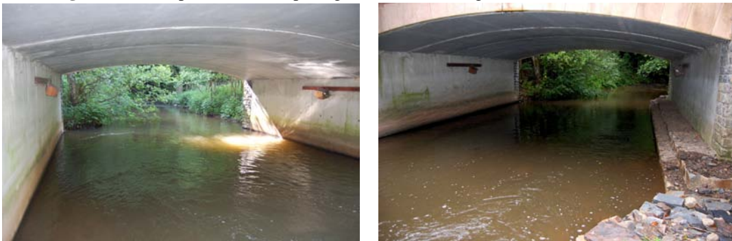
Figure 13. Example of a local stone passage under a bridge along the Wark River (Welscheid) (before and after the work)
