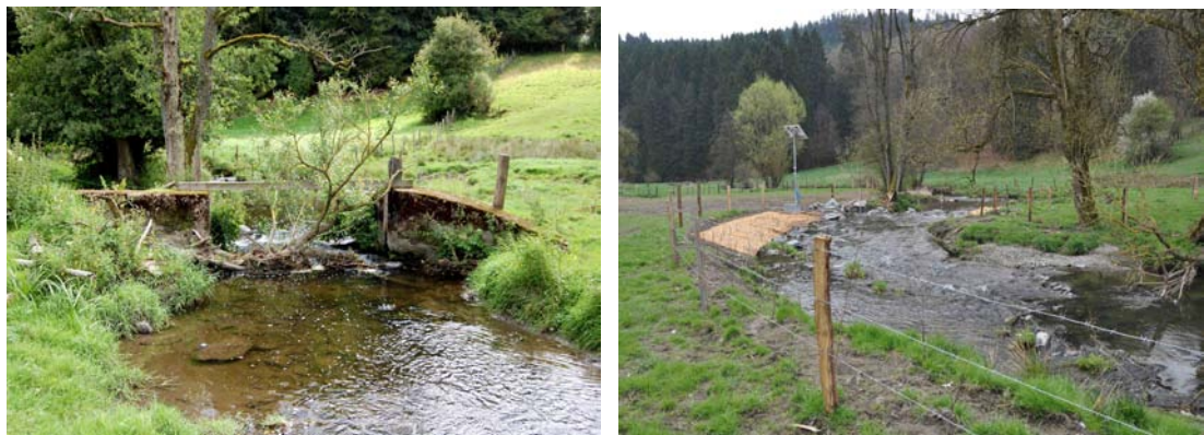
Figure 10. The removal of a concrete obstacle on the Wiltz River (before and after the work).
